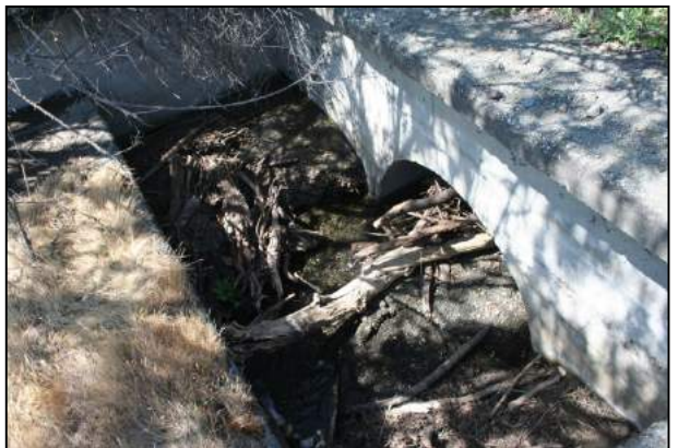
Figure 19: Hwy 101 Culvert 21 full of debris.
