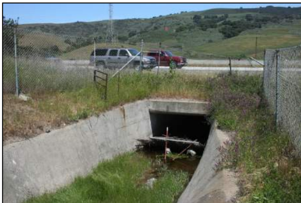
Figure 18: Hwy 101 Culvert 23 blocked by fence.
